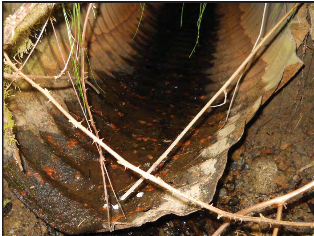
Culvert outlet - extensive rust and minor perforations forming.
