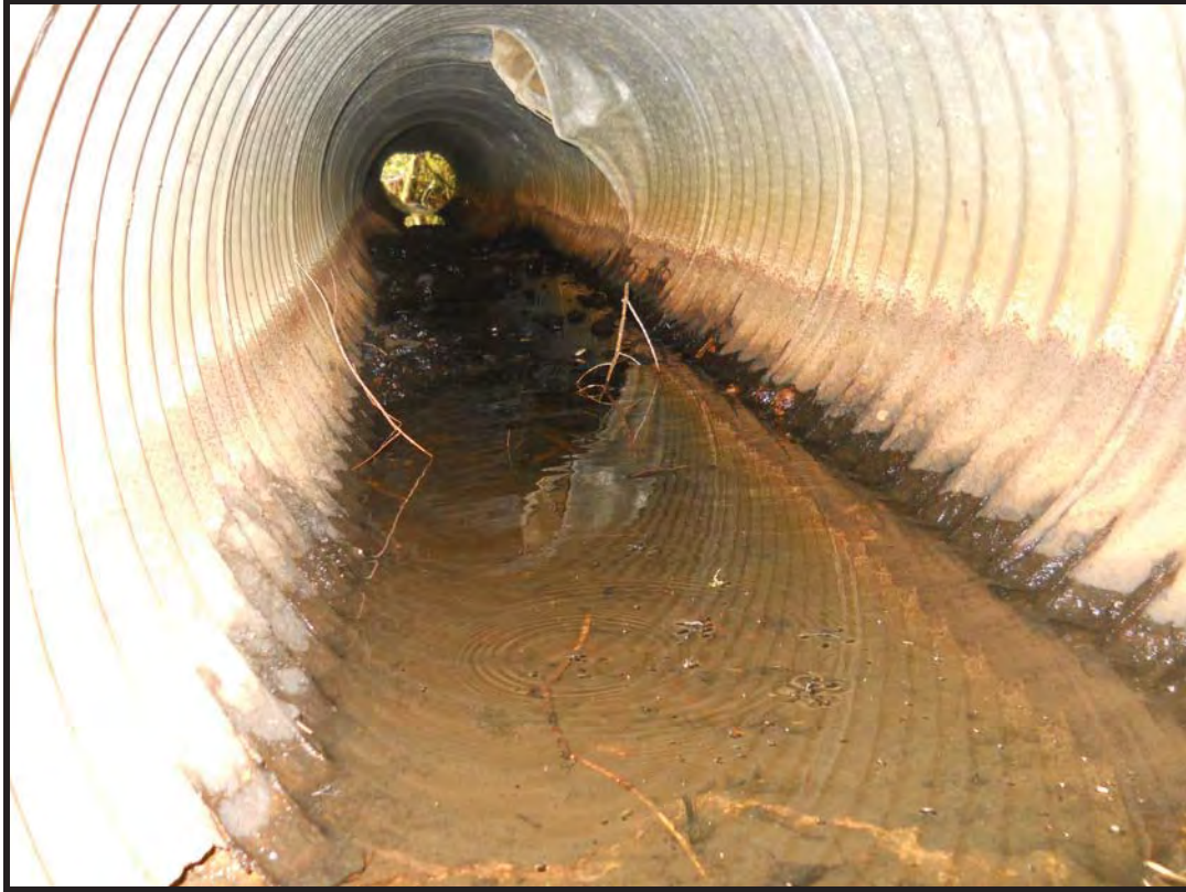
Culvert barrel at inlet - bottom rusted through and joint failure.
