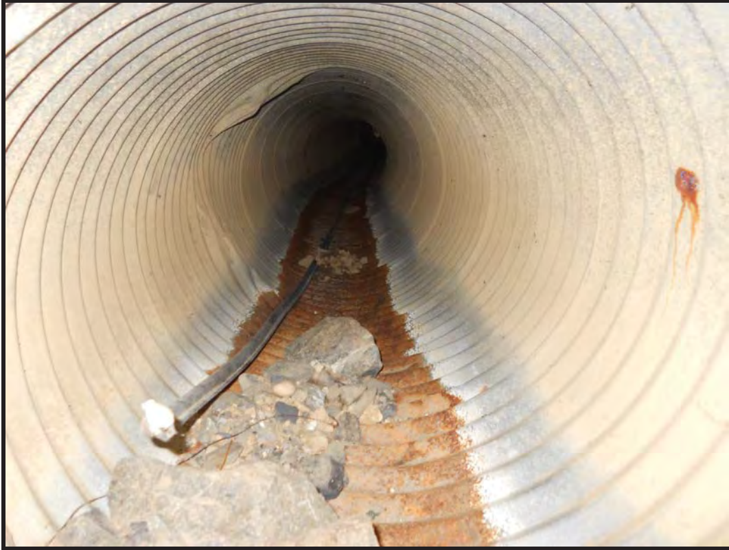
Culvert barrel at inlet – extensive rust, (perforations not visible in picture).
