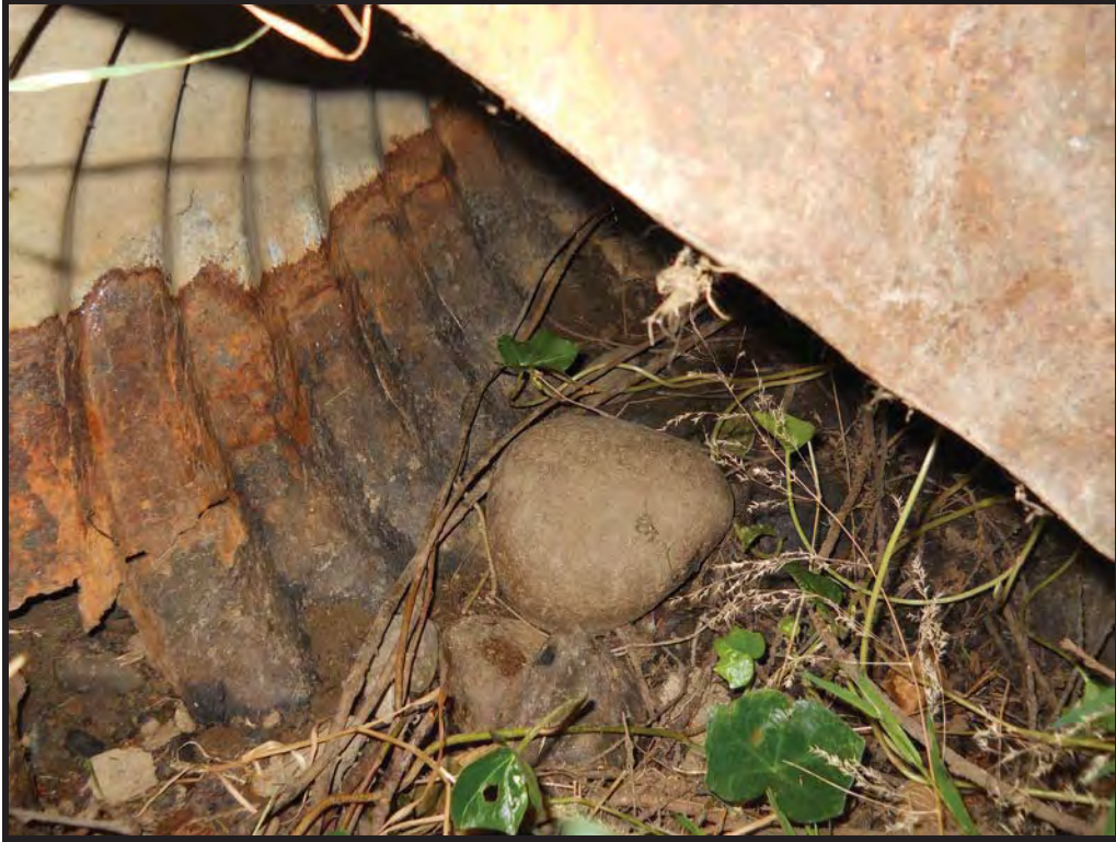
Culvert outlet - extensive rust and perforations.
