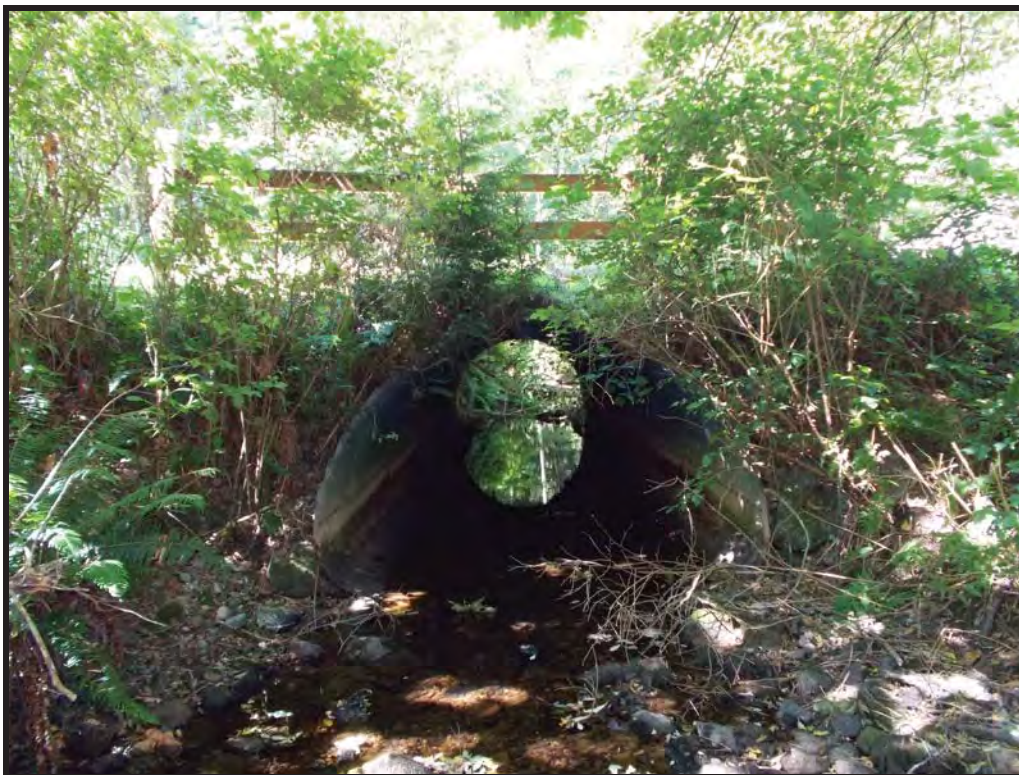
Culvert outlet – rust in bottom third of pipe
