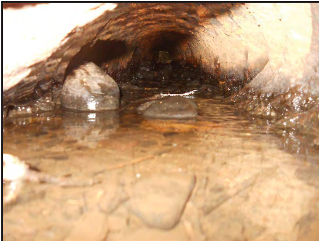
Culvert 408.2 outlet – extensive rust and sedimentation.
