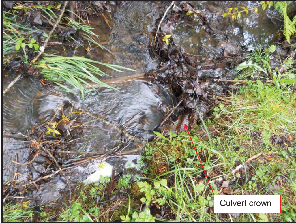
Culvert inlet - debris and channel backed up to crown of pipe.
