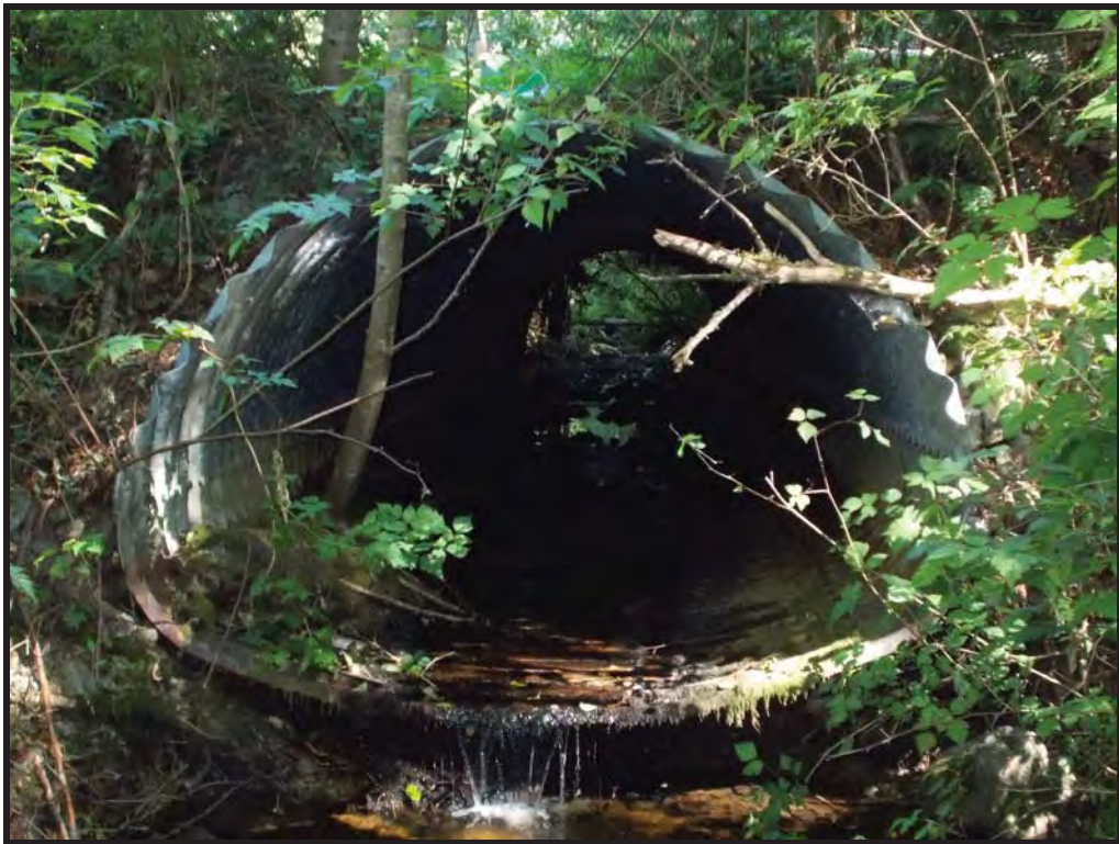
Culvert outlet – Hydraulic drop and scour undermining outlet.
