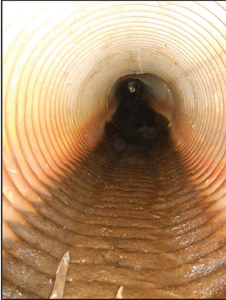
Culvert barrel at inlet - extensive rust, joint separation, pipe settlement.
