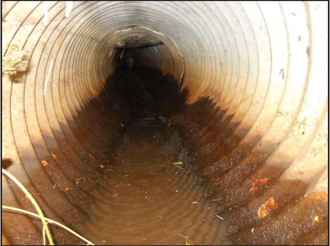
Culvert inlet - rust, joint separation and conflicting conduit/pipe.
