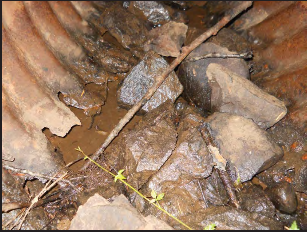
Culvert inlet – bottom rusted through.
