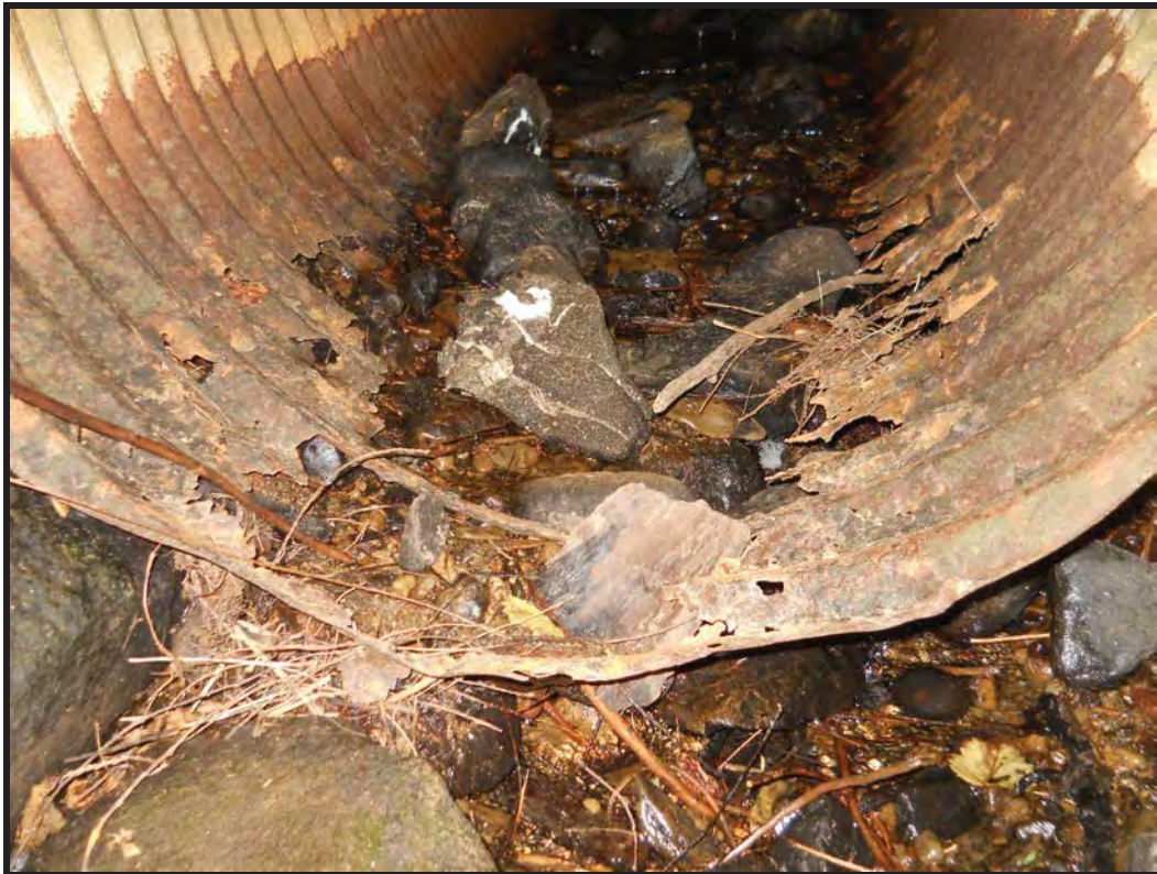
Culvert outlet – bottom completely rusted through
