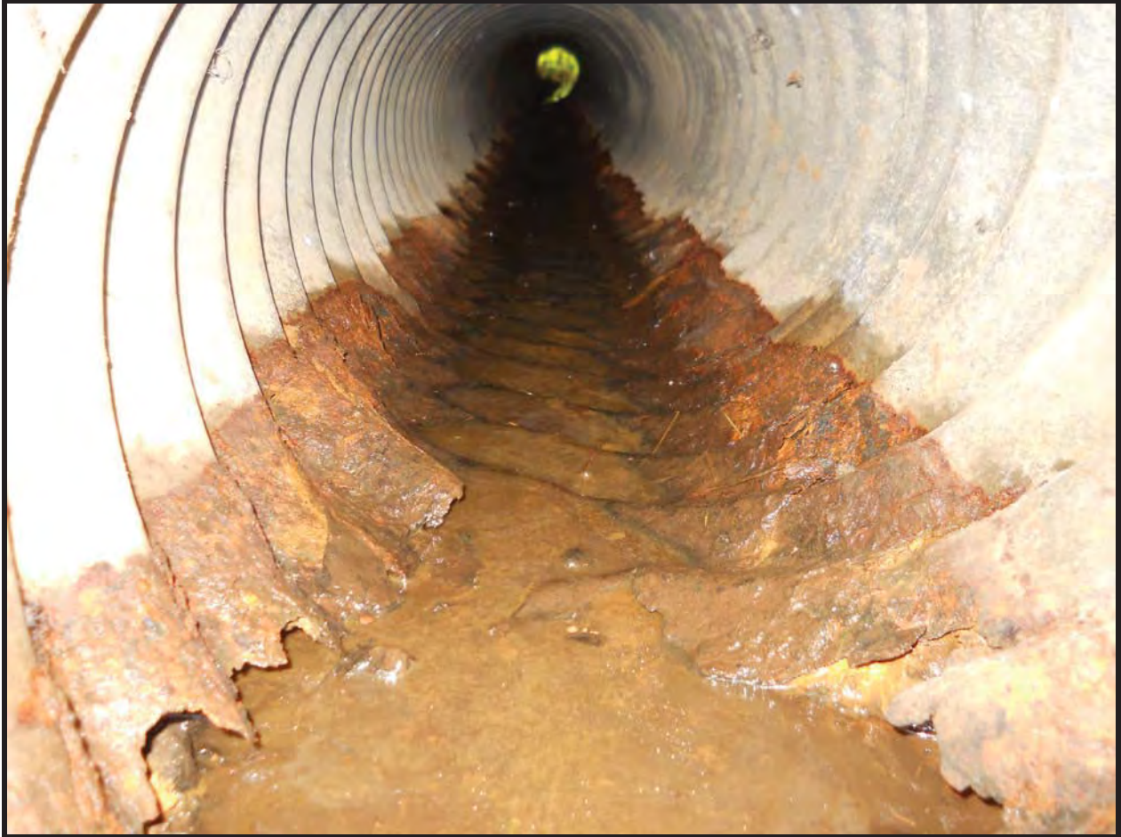
Culvert inlet showing rust through bottom.
