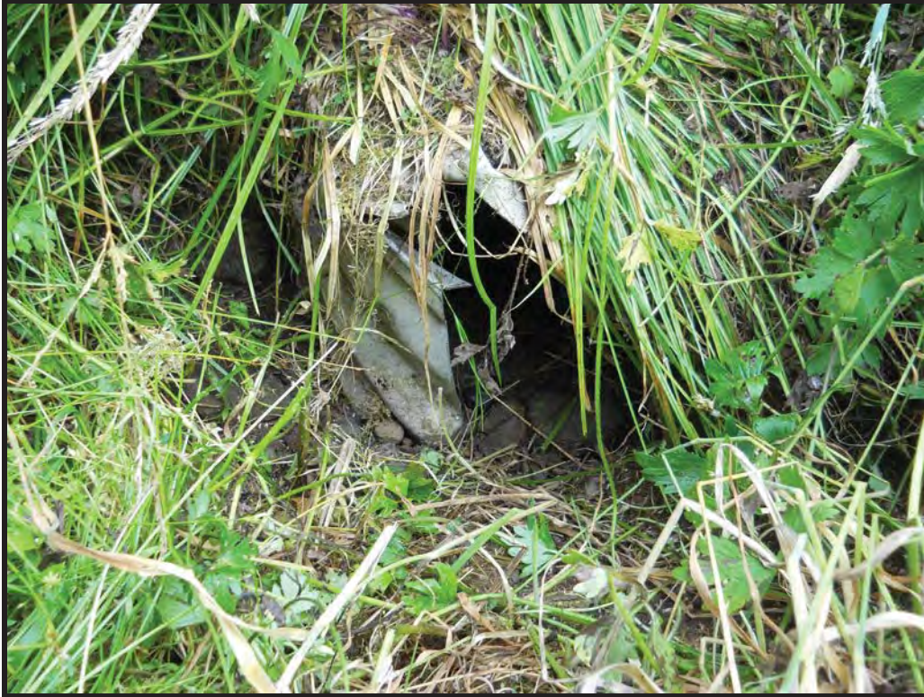
Crushed culvert inlet.
