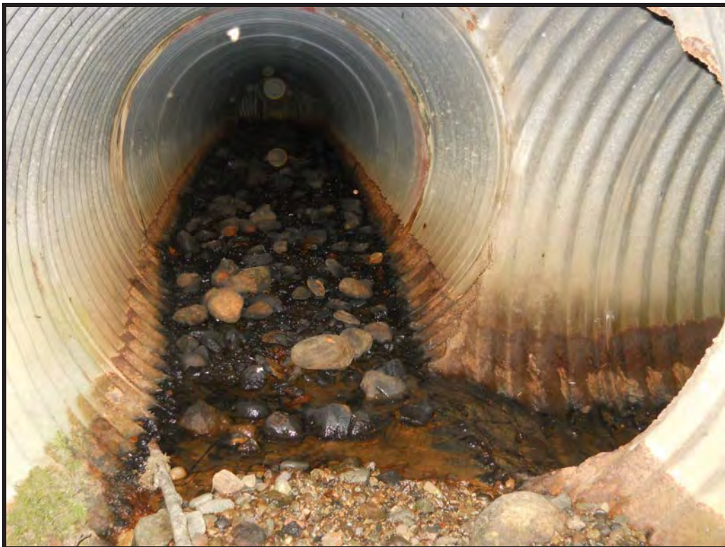
Junction of culverts 129, 130, and 131 – visible rust perforations, joint separation.
