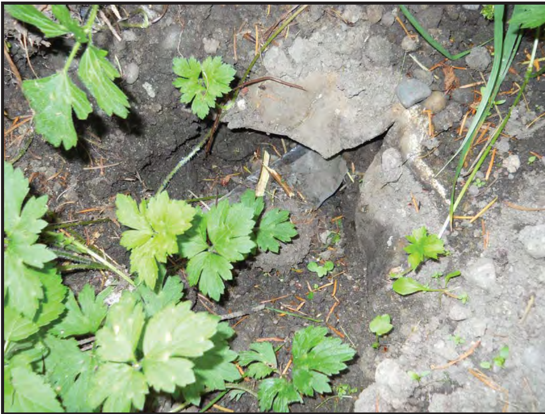
Crushed culvert outlet.
