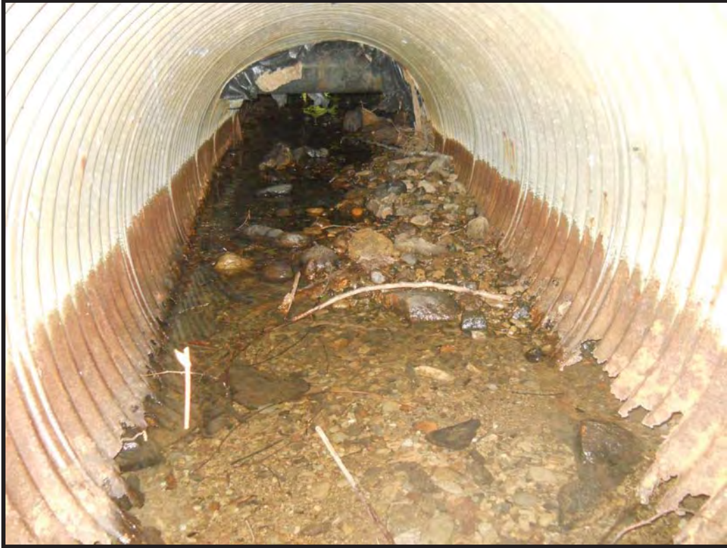
Culvert barrel at inlet - no bottom and conflicting sanitary sewer pipe.
