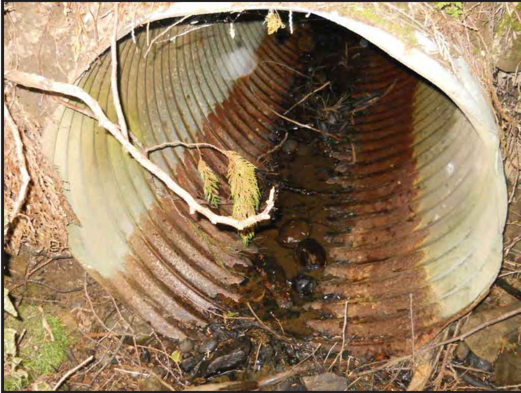
Culvert inlet - extensive rust, bottom disintegrated.
