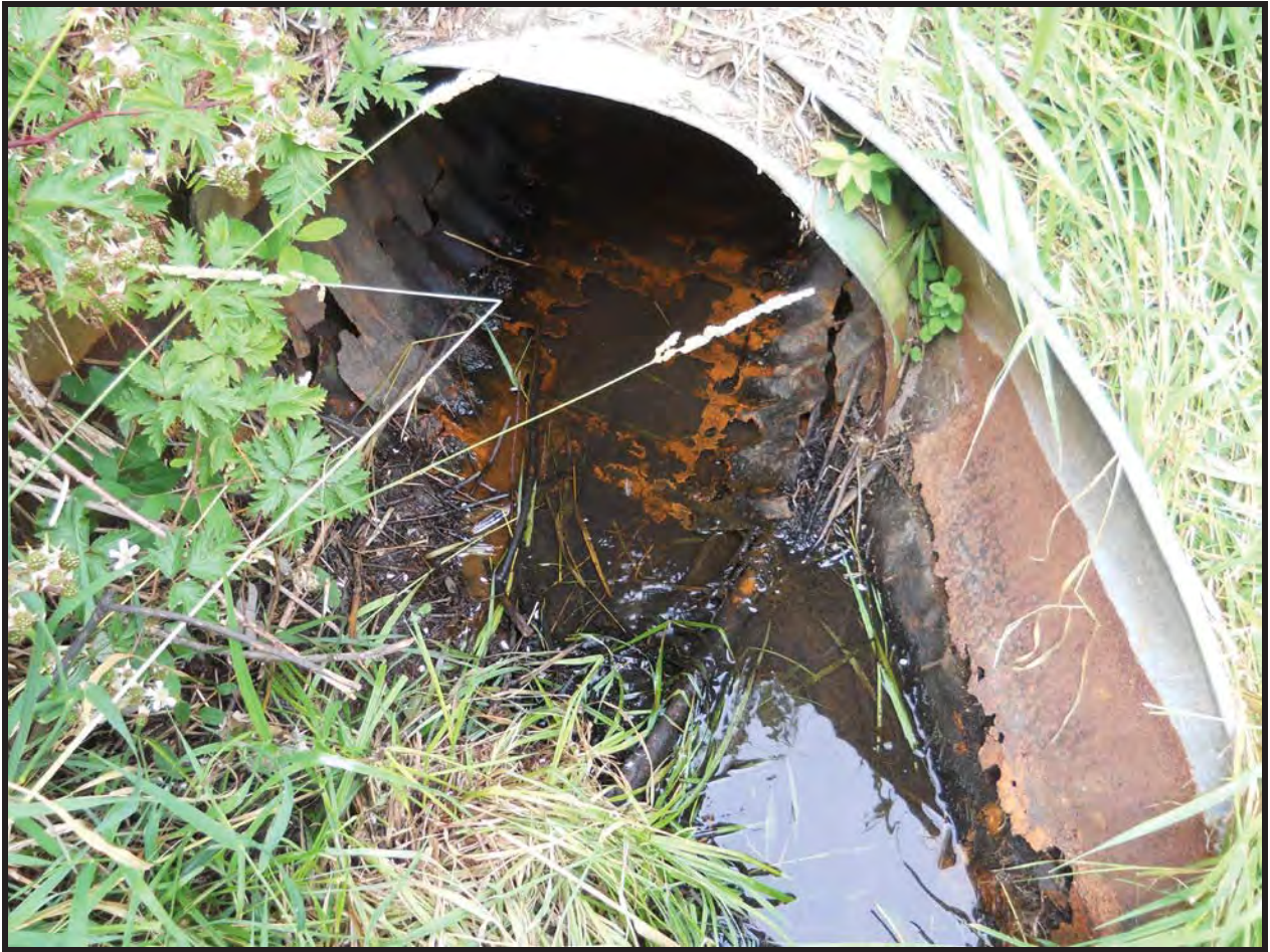
Culvert inlet extensive rust through.
