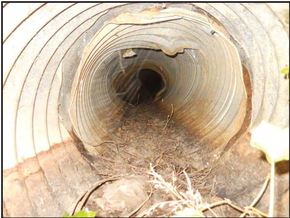
Culvert barrel at outlet - extensive settlement and joint separation.
