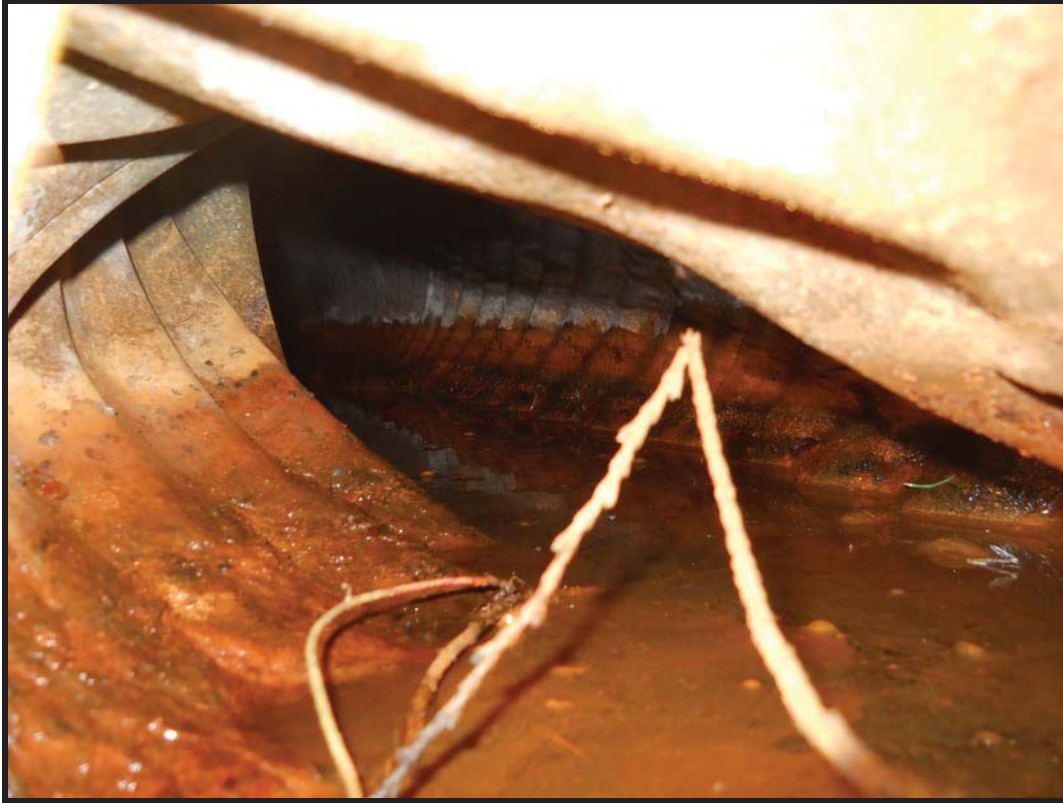
Culvert 408.1 inlet – extensive rust.
