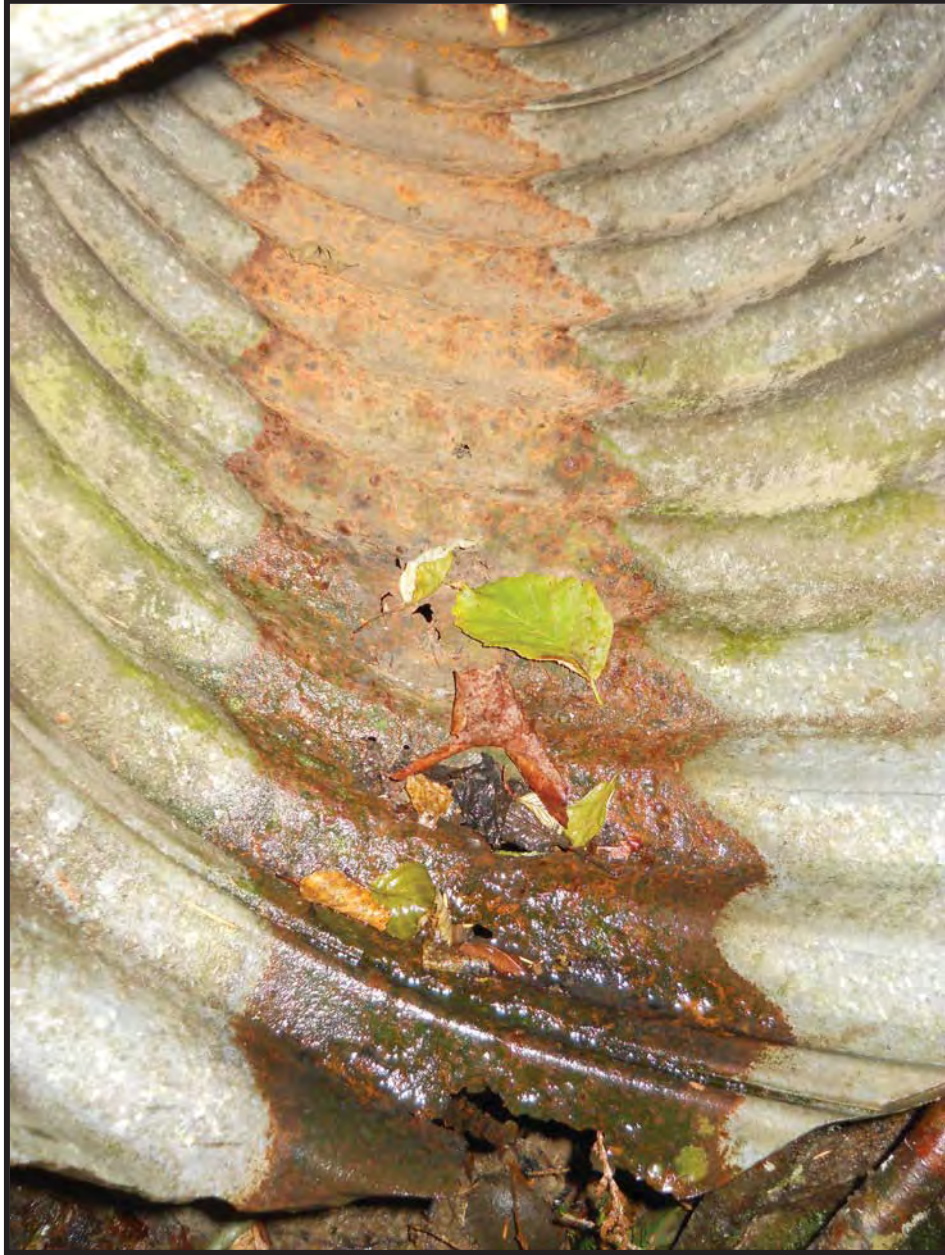
Culvert outlet – rust and perforations forming through bottom.
