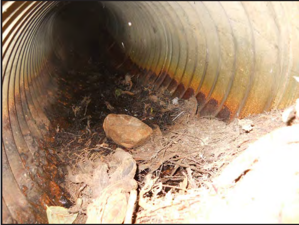
Culvert inlet - significant bottom rust and debris and tree roots.
