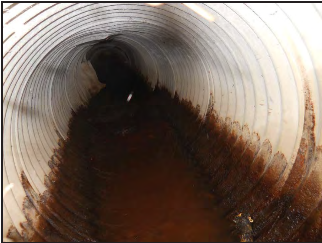
Culvert barrel at inlet (low flow) - extensive rust and joint separation/caving.
