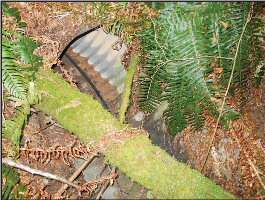
Culvert outlet - extensive rust, downstream channel de-stabilized.
