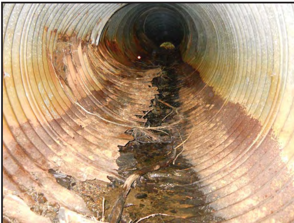
Culvert outlet – bottom disintegrated, joint separation, pipe settlement.
