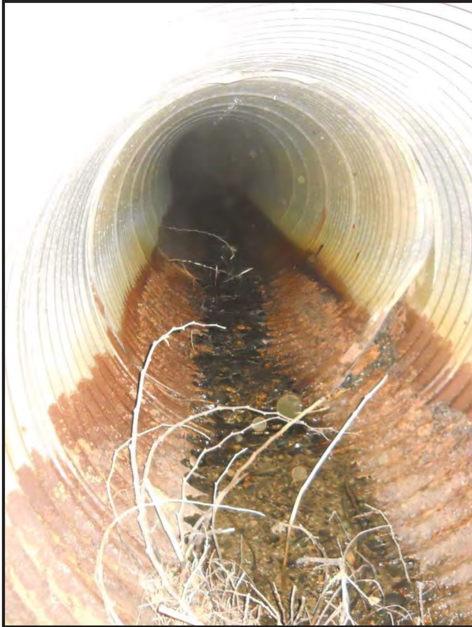
Culver barrel at inlet - bottom rusted through with joint separation.
