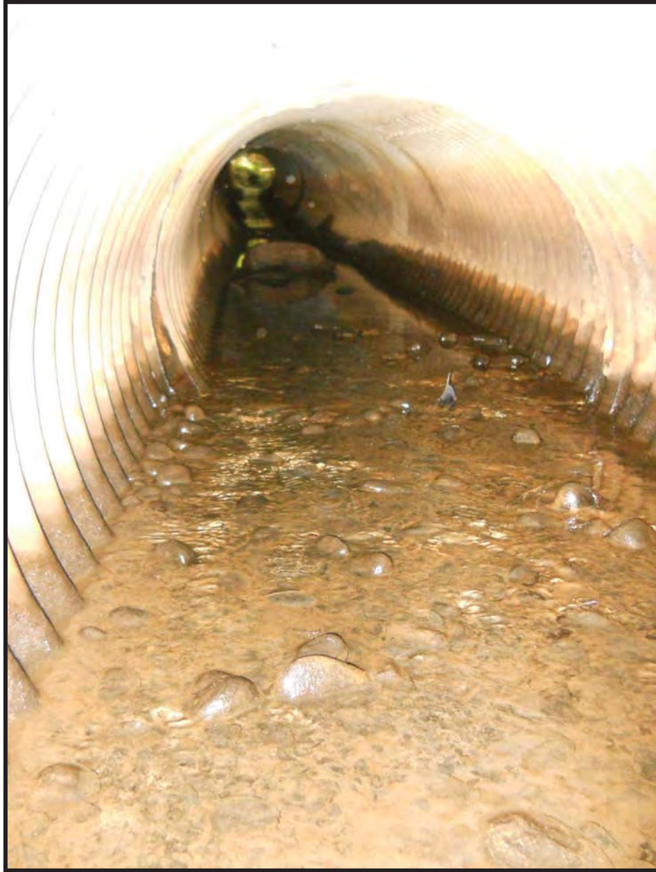
Culvert barrel at outlet – extensive rust, bottom disintegrated.
