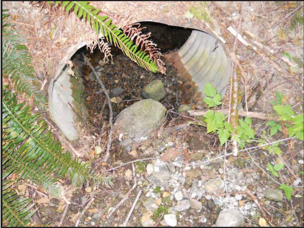
Inlet of Culvert 130 - pipe bottom disintegrated.
