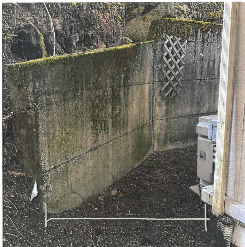
This is the left side of house (from street), gate will be connected to retaining wall.
