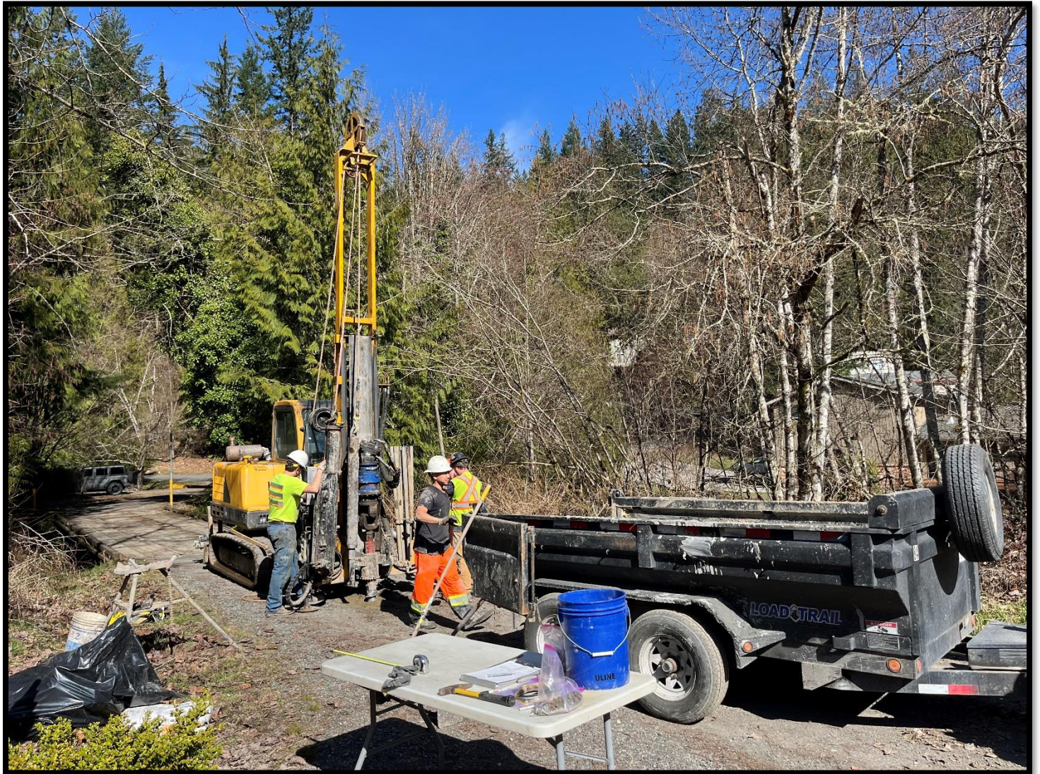
Photo 4: Facing north at borehole B-4 on the south side of Beaver Creek at Area Z on March 18, 2024.
