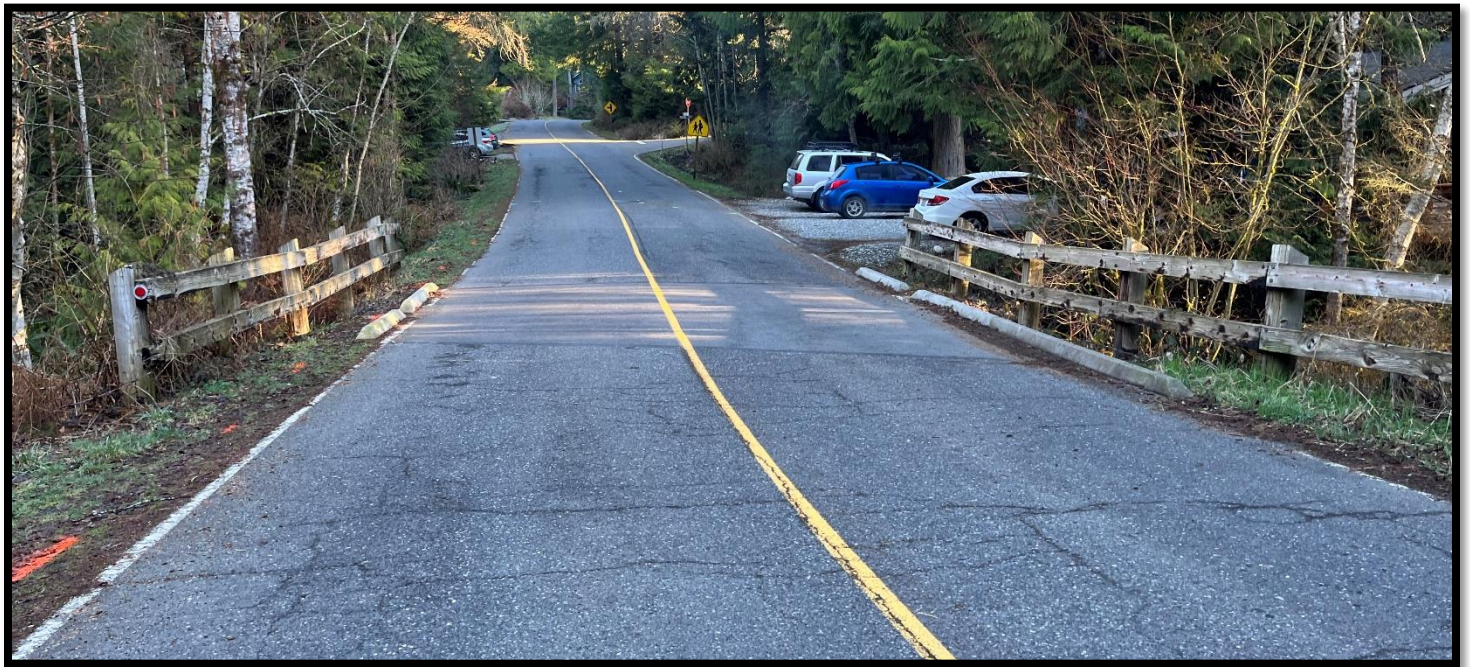
Photo 1: Existing conditions facing north on Polo Park Drive looking at the culvert crossing at Beaver Creek on March 18, 2024.
