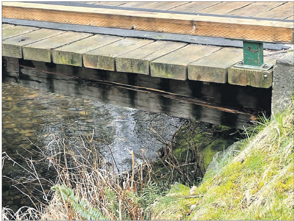
On Feb. 12, the SVCA Board of Directors approved the allocation of $56,243 from the Capital Repair and Replacement Reserve Fund, also known as CRRRF, for what Sudden Valley General Manager Jo Anne Jensen called “urgent repairs” to the course’s No. 1 and No. 4 bridges. Pictured is bridge No. 4. (SVCA photo)
