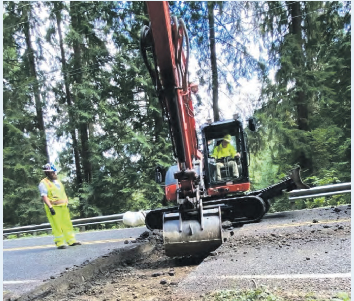
Whatcom County Public Works issued an Emergency 24/7 closure of Lake Whatcom Blvd. between Lake Louise Road and Southern Court beginning Monday, Sept. 18 to replace a failing culvert that was causing severe shoulder erosion. Lake Whatcom Blvd. was reopened for travel on the afternoon of Sept. 21. (Photos courtesy Whatcom County Public Works)
